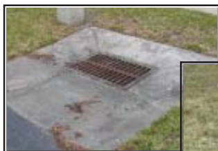
Catch basin w/collar
